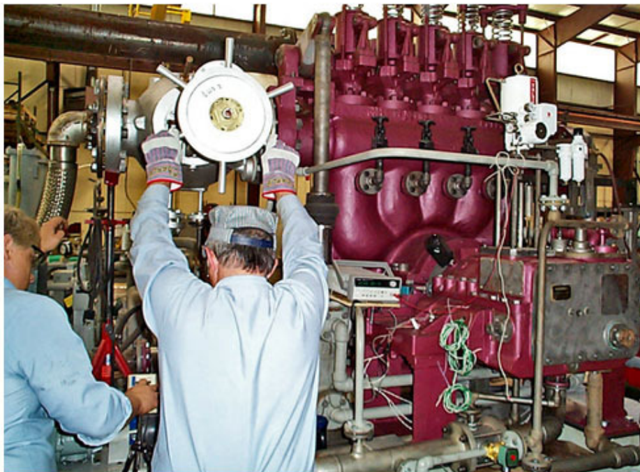
Baltimore Refuse Energy Company—turbine generator installed by Turbosteam in Baltimore, MD
